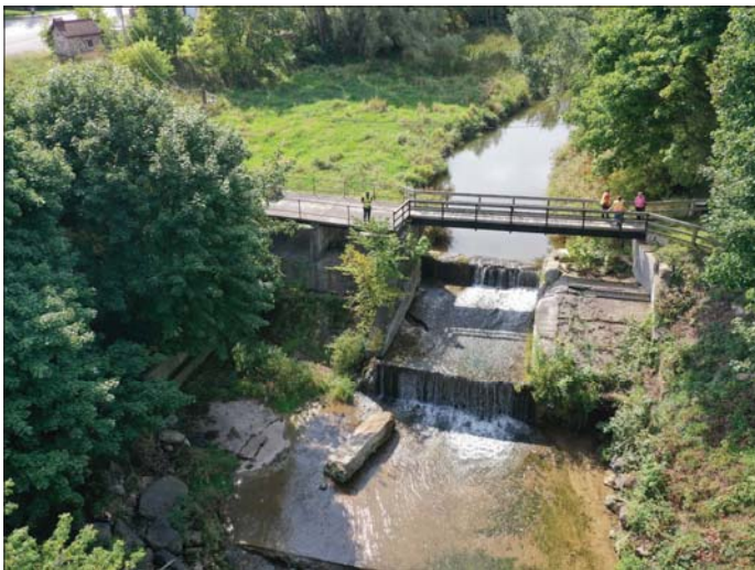
Photo 27 - September 20, 2022 Neustadt Dam and Flood Control Wall Aerial View of Downstream Side of Dam
