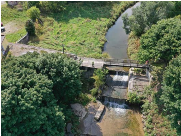
Photo 51 - September 20, 2022 Neustadt Dam and Flood Control Wall Aerial View of Downstream Side of Dam
