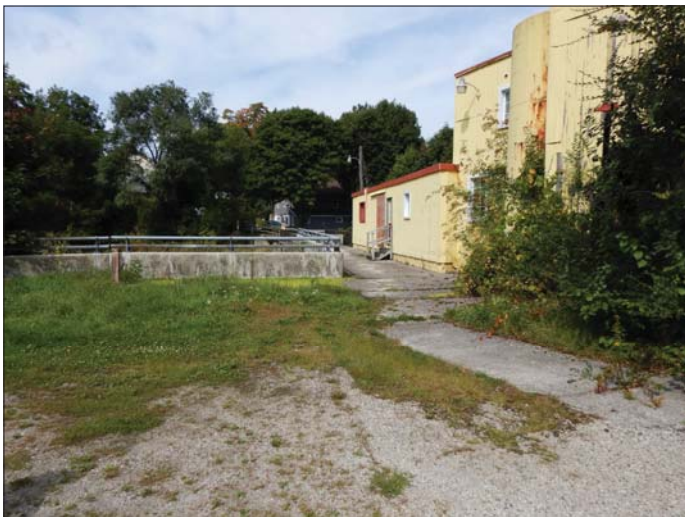
Photo 39 - September 20, 2022 Neustadt Dam and Flood Control Wall Left Side of Dam and Flood Control Wall
