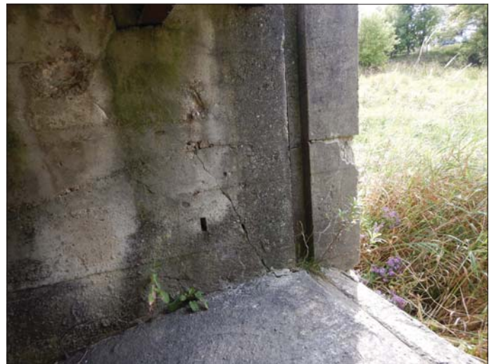
Photo 10 - September 20, 2022 Neustadt Dam and Flood Control Wall Control Structure, Sluice 1 Left Gain
