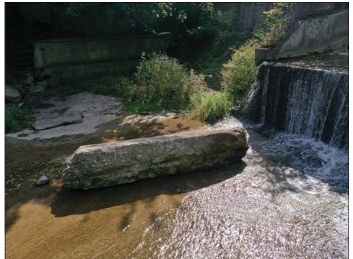
Photo 30 - September 20, 2022 Neustadt Dam and Flood Control Wall Downstream Left Side of Dam
