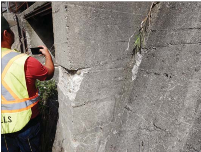
Photo 9 - September 20, 2022 Neustadt Dam and Flood Control Wall Upstream Side of Control Structure, Sluice 1
