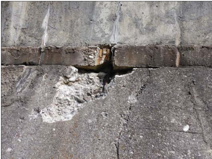
Photo 7 - September 20, 2022 Neustadt Dam and Flood Control Wall Upstream Side of Flood Control Wall
