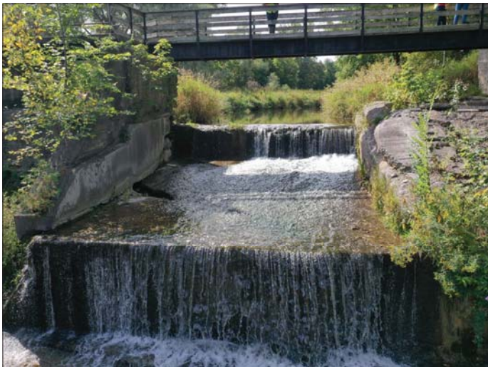
Photo 29 - September 20, 2022 Neustadt Dam and Flood Control Wall Downstream Side of Weir Structure
