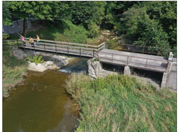
Photo 26 - September 20, 2022 Neustadt Dam and Flood Control Wall Aerial View of Upstream Side of Dam
