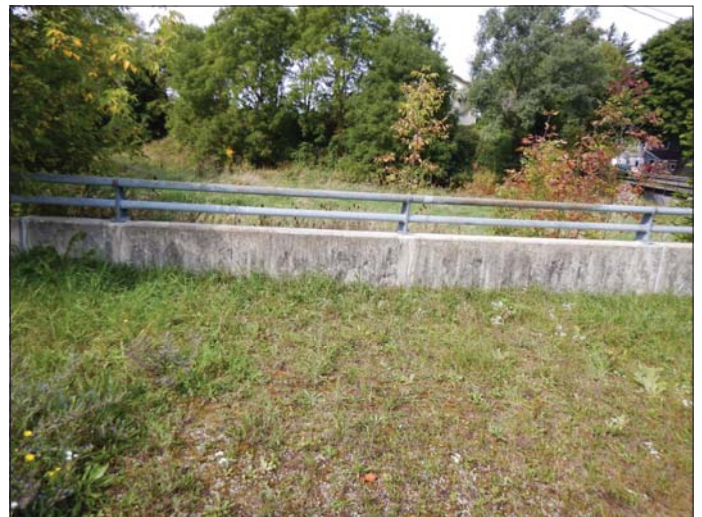
Photo 40 - September 20, 2022 Neustadt Dam and Flood Control Wall Back of Flood Control Wall
