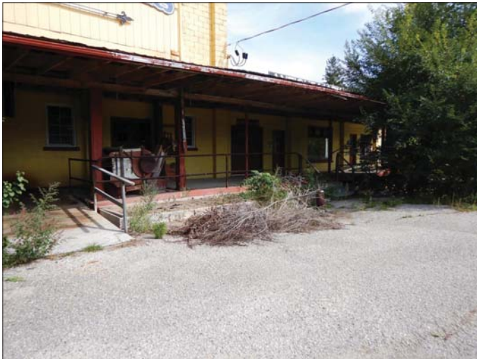
Photo 37 - September 20, 2022 Neustadt Dam and Flood Control Wall Building on Left Side of Dam
