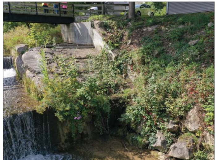
Photo 28 - September 20, 2022 Neustadt Dam and Flood Control Wall Downstream Right Side of Dam
