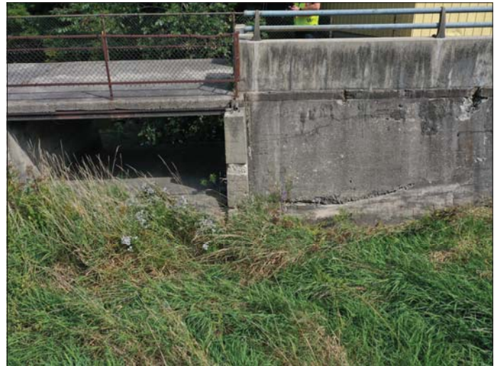
Photo 8 - September 20, 2022 Neustadt Dam and Flood Control Wall Upstream Side of Control Structure, Sluice 1
