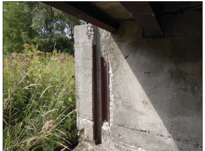
Photo 12 - September 20, 2022 Neustadt Dam and Flood Control Wall Control Structure, Sluice 1 Right Gain
