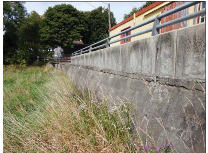
Photo 6 - September 20, 2022 Neustadt Dam and Flood Control Wall Upstream Side of Flood Control Wall
