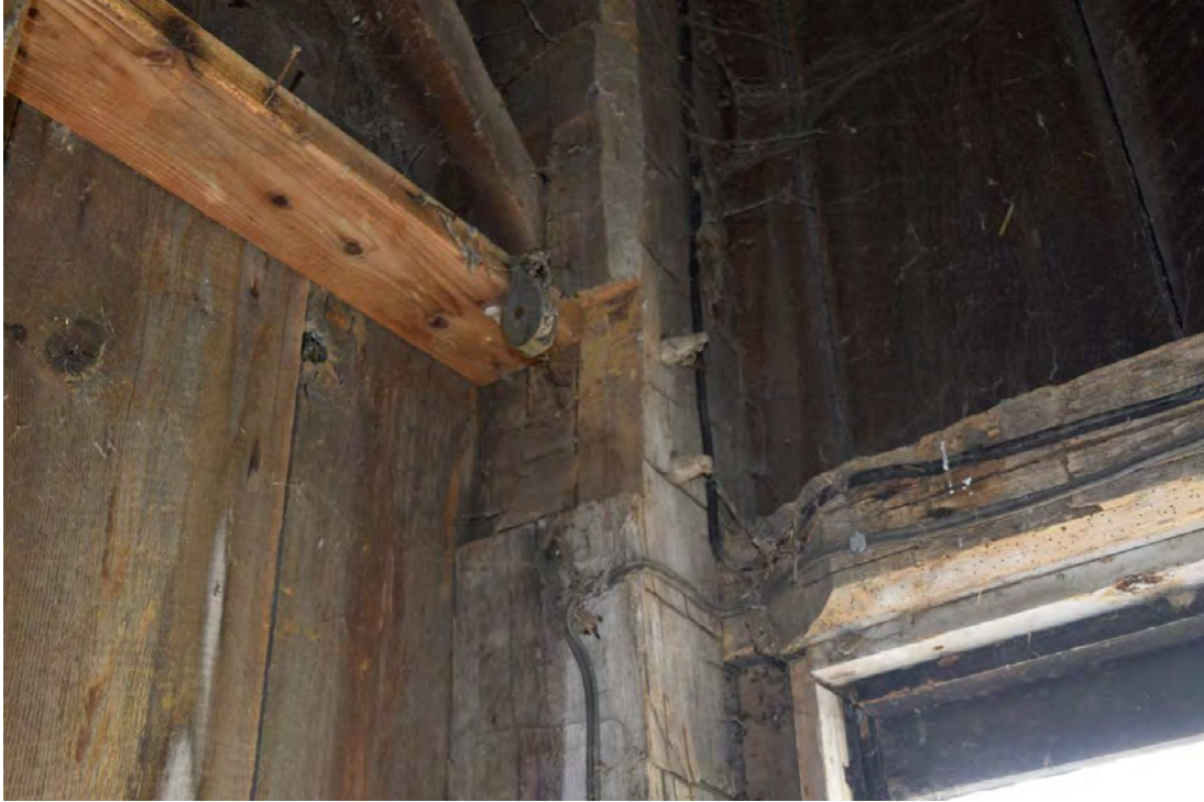
FIGURE 47: EXAMPLE OF TYPICAL USE OF HAND HEWN TIMBER FRAME COMPONENTS MIXED WITH MODERN DIMENSIONAL LUMBER
