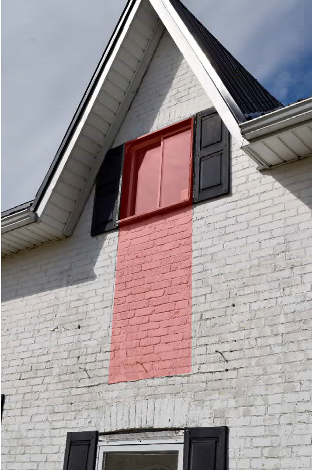
FIGURE 19: ALTERATION OF ORIGINAL STRUCTURAL OPENING IN CENTER GABLE, LIKELY A DOOR OPENING THAT WAS ALTERED TO ACCEPT A WINDOW, HIGHLIGHTED IN RED
