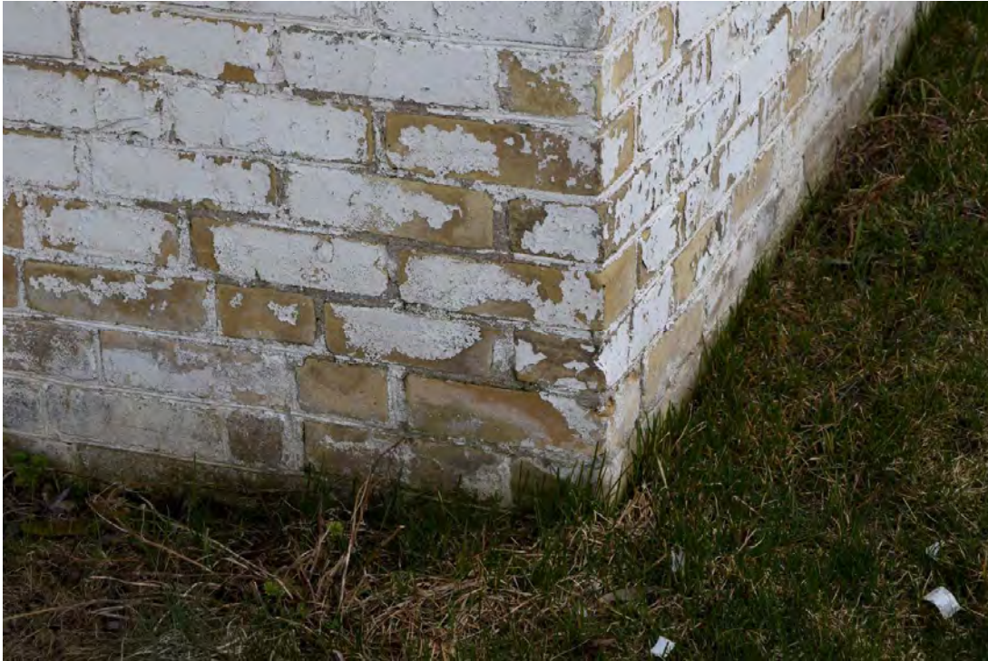
FIGURE 21: ORIGINAL YELLOW BRICK UNDER PEELING WHITE PAINT
