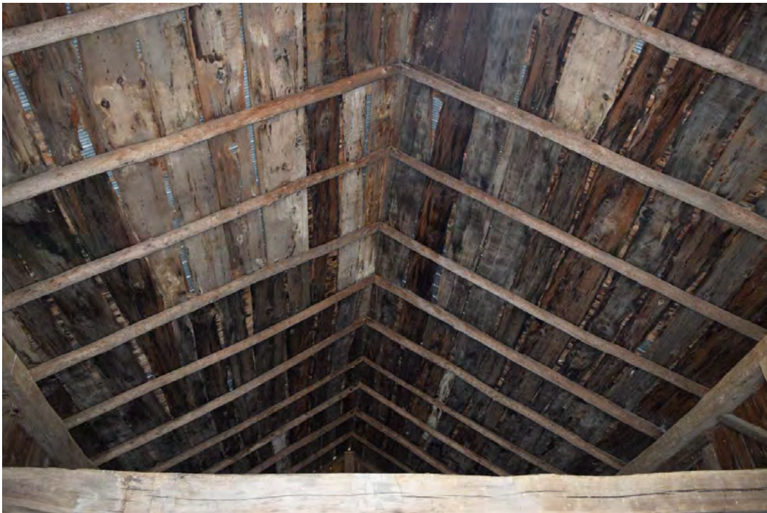
FIGURE 30: ROOF STRUCTURE OF SMALLER TIMBER FRAME STRUCTURE, NOTE RAFTERS ARE IN THE ROUND AND THERE IS NO RIDGE BEAM, TYPICAL OF EARLY CONSTRUCTION PRACTICES
