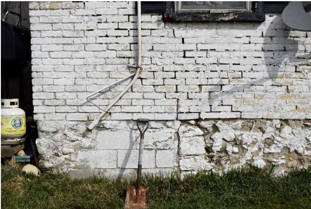
FIGURE 16: EVIDENCE OF MODIFICATION TO FOUNDATION
