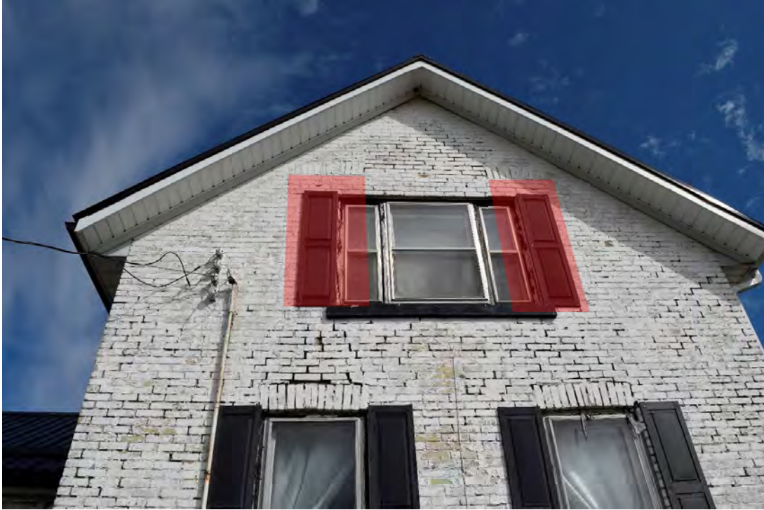
FIGURE 15: MODIFIED WINDOW OPENINGS ON SECOND STOREY OF SOUTH FACE, RED INDICATES LOCATION OF ORIGINAL WINDOW OPENINGS, NOTE THE OPEN MORTAR JOINTS BETWEEN BRICKS
