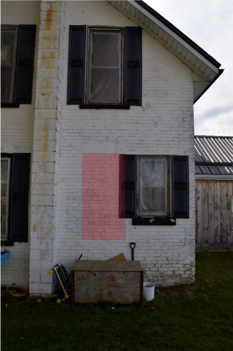
FIGURE 20: ALTERED WINDOW OPENING ON FIRST FLOOR OF NORTH FACE, ORIGINAL OPENING HIGHLIGHTED IN RED
