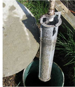
Clogged effluent filters can lead to sewage back ups.
