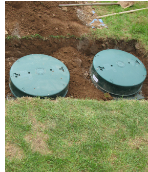
Tank risers ensure safety and accessibility for servicing.
